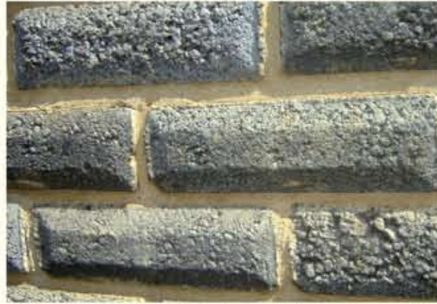
If the brick-work is flush jointed or the mortar has been pointed, it is not necessary to perform the previous step
