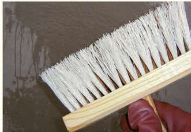
Wet the coated walls 3 times during the next day using clean water
